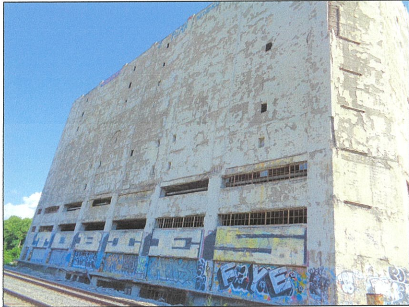
Photograph 7 -August 1 st , 2022 (Completed -Task 2 removal of all loose & failing masonry along the Southerly face of the building)
