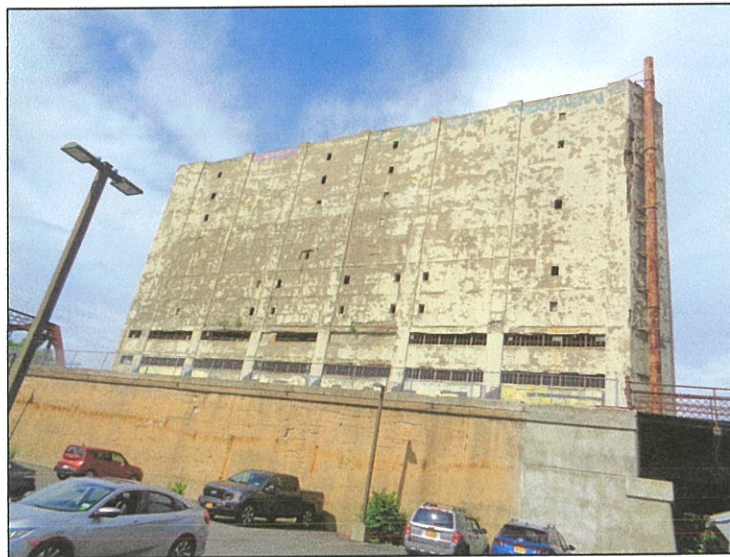
Photograph 1 (Photo taken July 26 th , 2022) (South exterior wall-Central Warehouse building prior to implementing emergency remediation measures)
