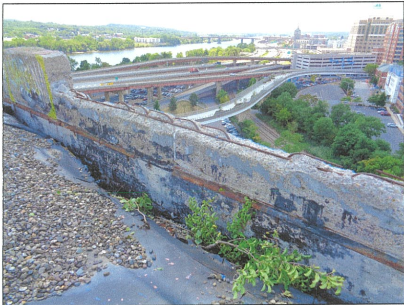
Photograph 8 -August 1 st , 2022 (Completed -Task 3 removal of all loose & failing masonry along the Southerly parapet wall)
